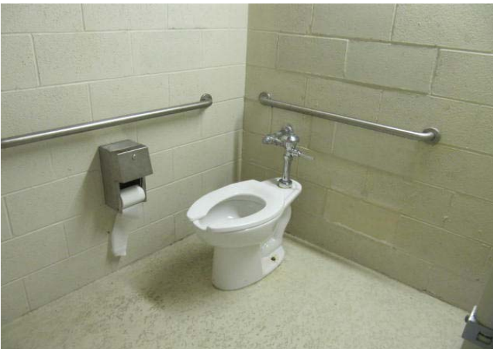
Toilet and wall-mounted ADA grab bars at pool house.
