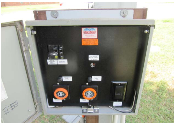
Timers, fuses, lighting switches, and breakers.
