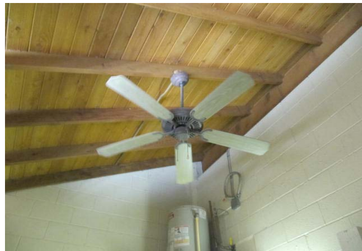
Ceiling fan at pool house interior.
