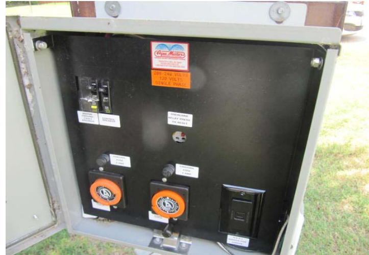
Control box / timer for pond aerator.
