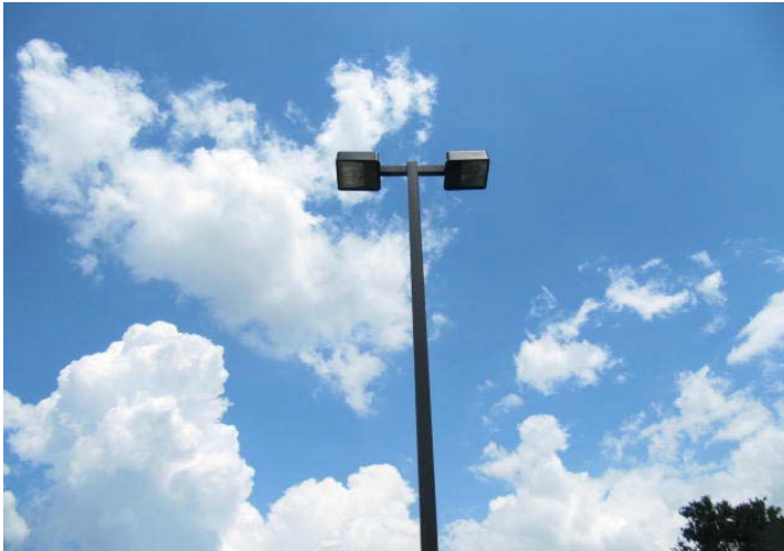
Overview of light pole and fixture at parking lot.
