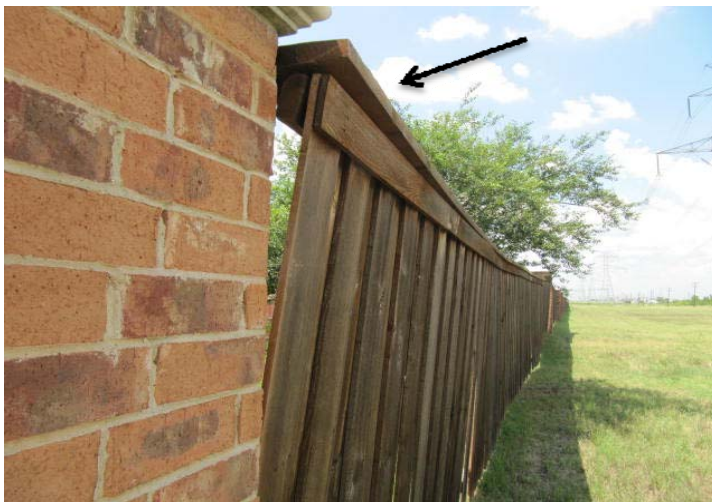
Isolated condition of detached fence section.
