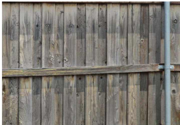
Wood privacy fence along transmission line easement.
