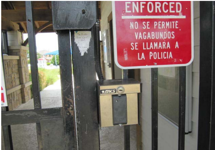
Overview of FOB access / proximity card reader.
