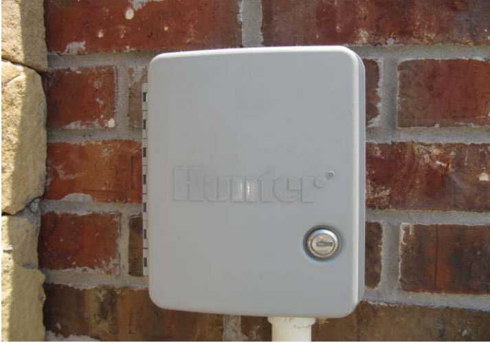
Irrigation controller / timer.
