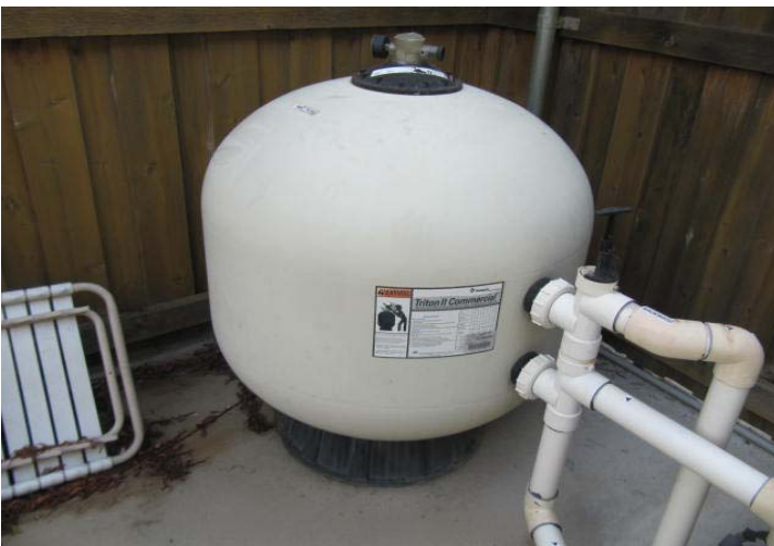
Typical sand filter at swimming pool.
