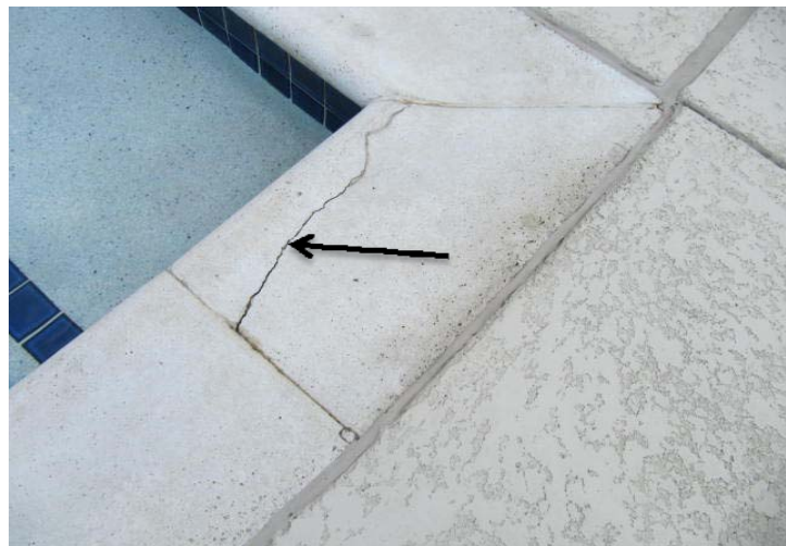
Cracked coping section at pool perimeter.
