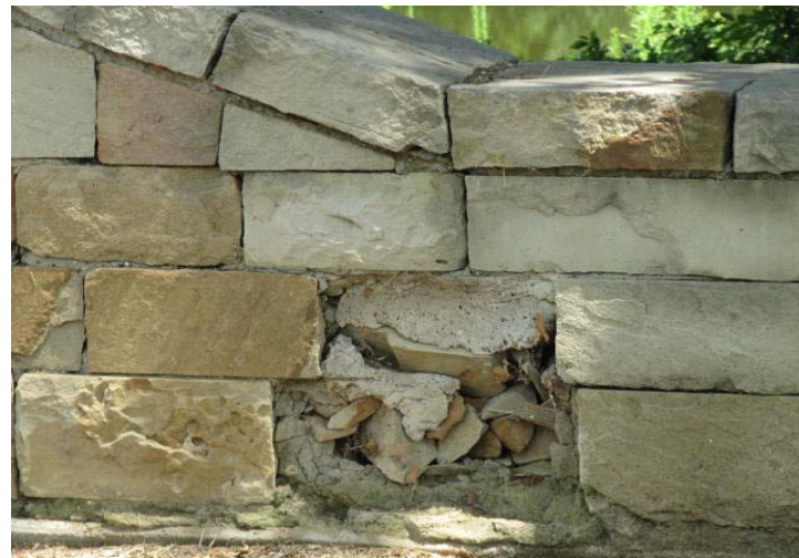
Damaged stone wall along entrance drive at Southwind Drive.
