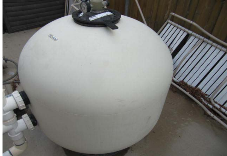
Typical sand filter at swimming pool.
