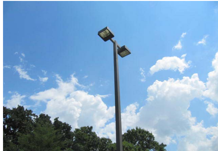
Duplex fixture at light pole.
