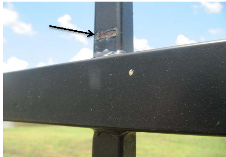
Isolated condition of worn finish & surface oxidation.
