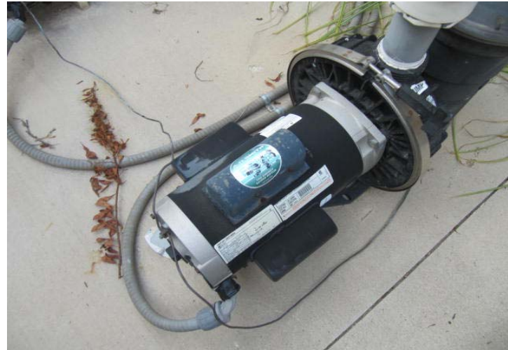
Circulating pump, at wood enclosure near pool house.
