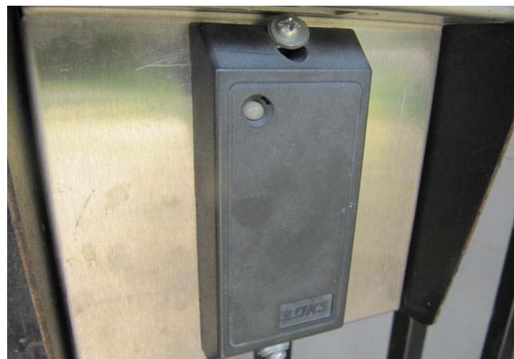
Close-up view of FOB access / proximity card reader.
