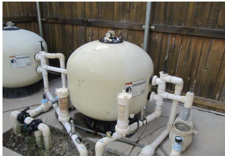
Original pool filter, in good functional condition.
