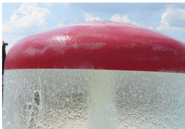
Good finishes at water feature - recent painting funded from operating budget.
