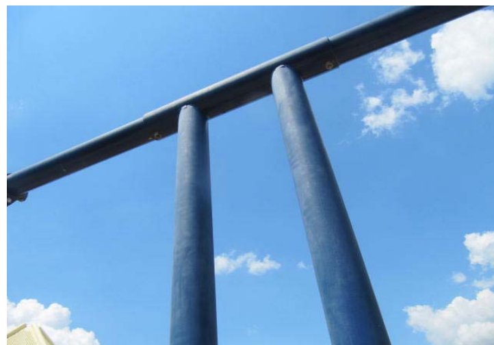
Worn finishes at swing set structure - fund paint finishes through operating budget.
