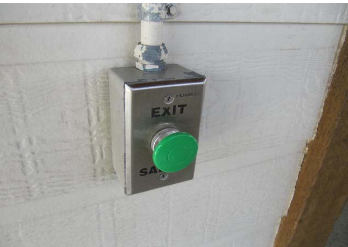
Gate release button at inside of pool gate.
