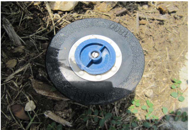
Irrigation sprinkler head at planting bed near monument sign.
