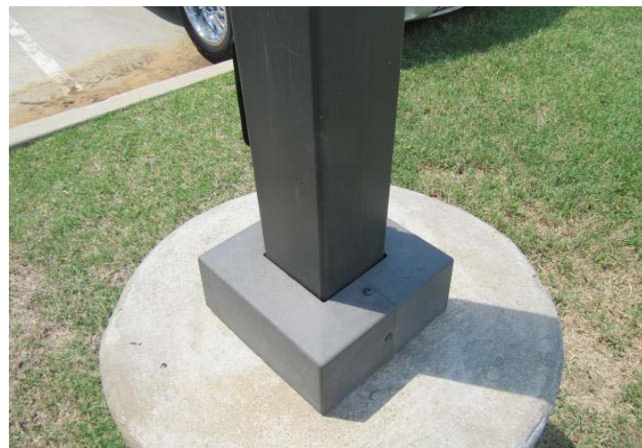
Aluminum base cover at light pole.
