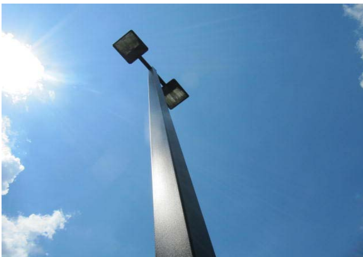
Duplex fixture at light pole.
