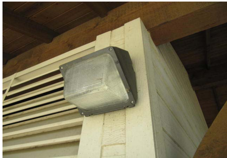
Wall mounted light fixture at pool house.
