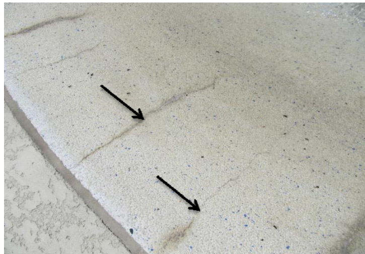
Cracks at pool finish near zero-depth area.
