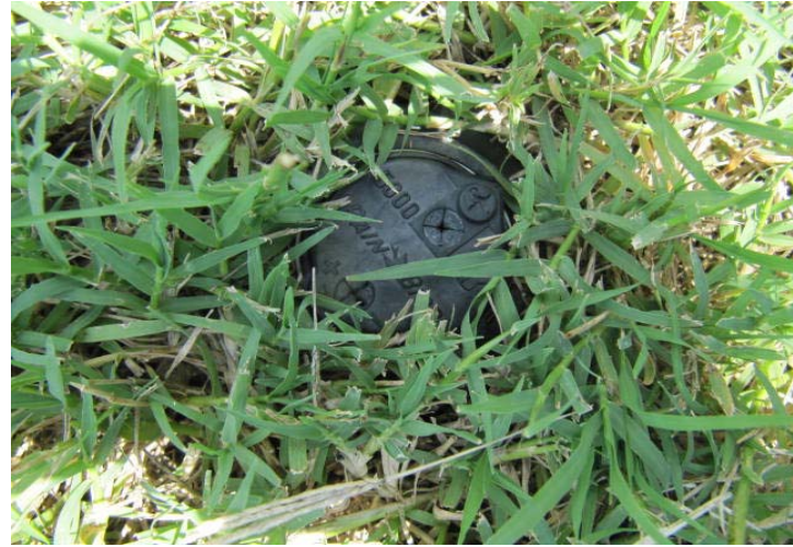
Irrigation sprinkler head at lawn area near pond.
