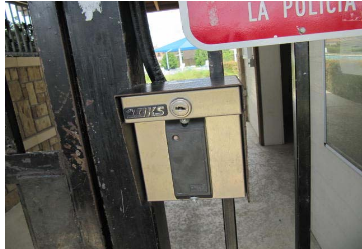
Overview of FOB access / proximity card reader.
