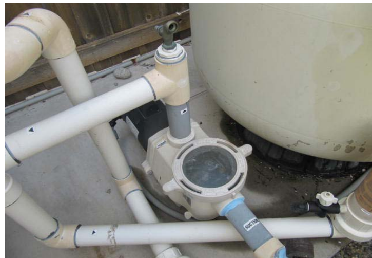
Pool circulating pump, in good functional condition.
