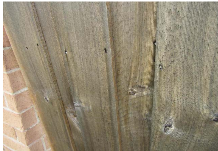
Typical condition at wood pickets at fence.
