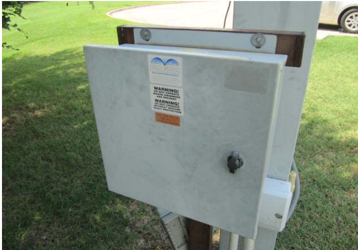
Overview of control box / timer.
