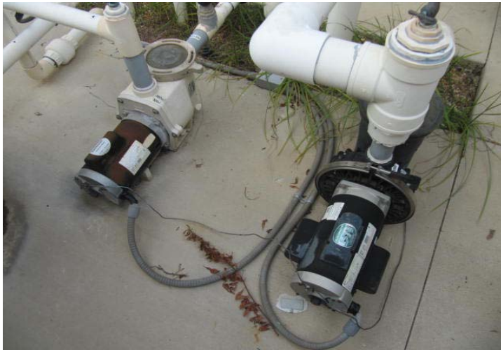
Circulating pumps for swimming pool.
