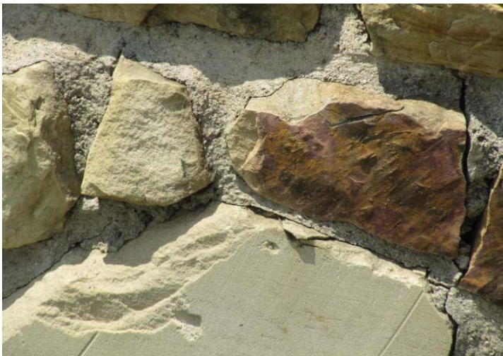
Cracked mortar joints at stone retaining wall.
