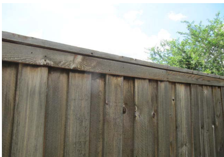
Typical shadow box style fence with top rail.
